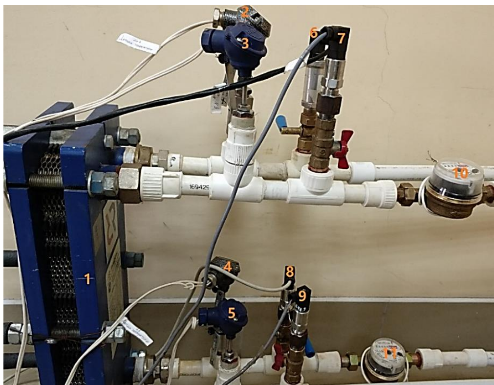
Figure 3. Experimental test section: 1 — plate heat exchanger; 2, 3, 4, 5 — M5100 pressure transmitters; 6, 7, 8, 9 — thermometers; 10, 11 — mechanical flow meters.
